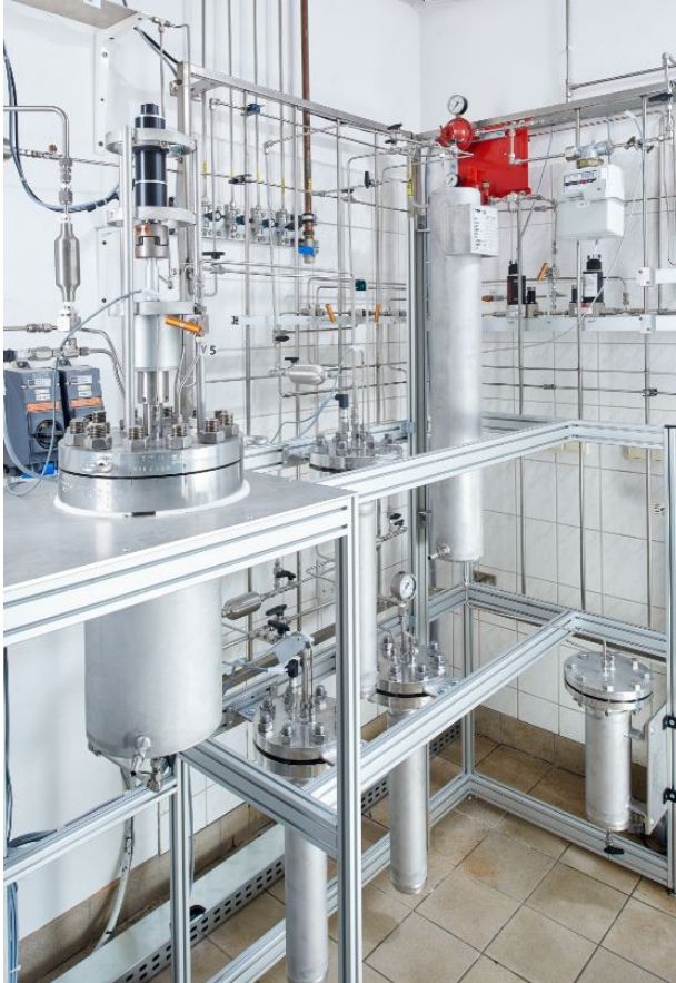
Fig.: EDL's expanded SDA pilot plant in Leipzig / Germany
